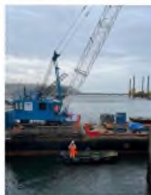
▲ Repair of the Sutton Harbour lock gates is now underway – but it is claimed that the 'mitigation measures' promised to displaced fishermen have not been forthcoming.
